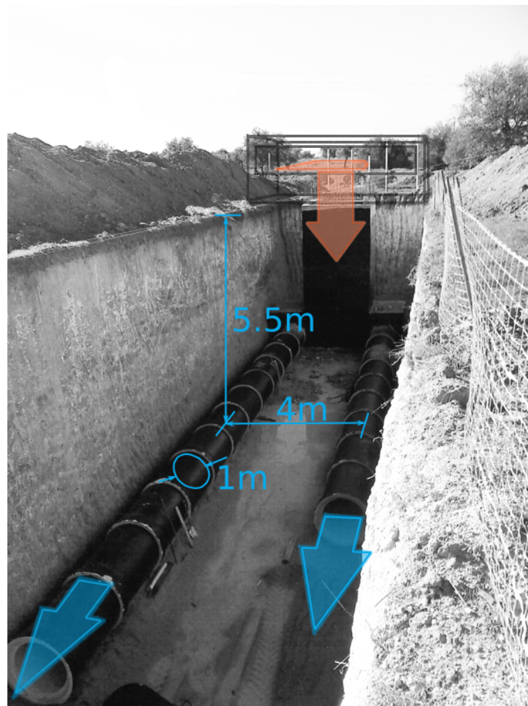
Figure 3. Photograph of the EAHX while the buried pipes were being installed at an average depth of 5.5 m below soil surface.
